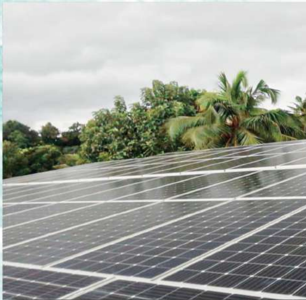
25 kW ON-GRID AT MAYA RESTAURANT, ETTUMANOOR
