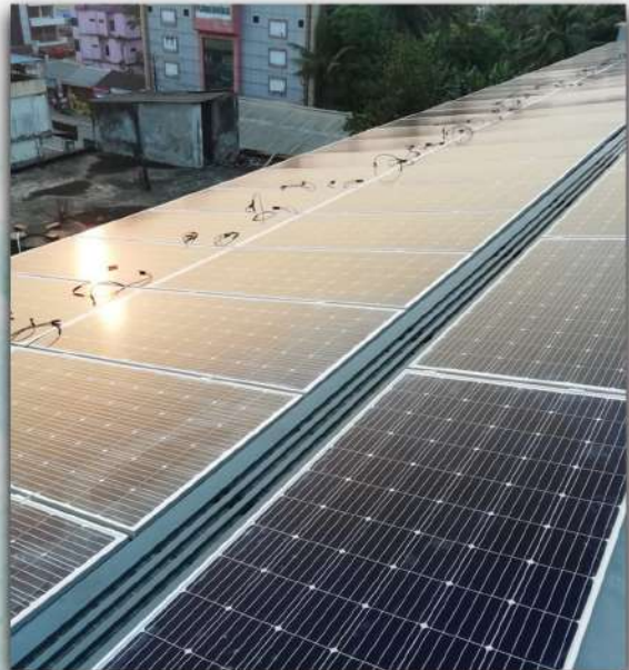
50 kW AT ELBA TRADERS , ETTUMANOOR (WHEELING)
