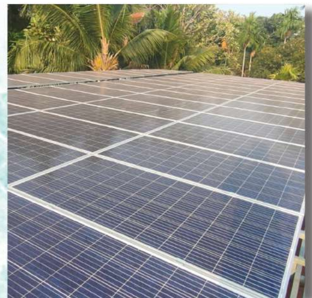
30 kW ON-GRID AT SIVAN & SONS MAVELIKARA
