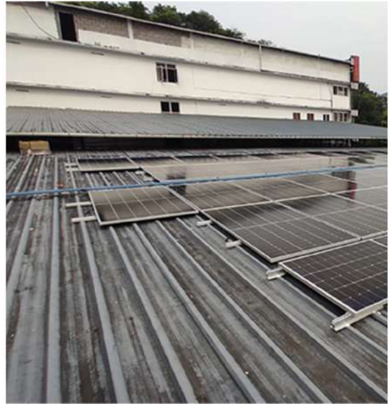
50 kW AT THOTTUNGAL TRADING COMPANY, IDUKKI
