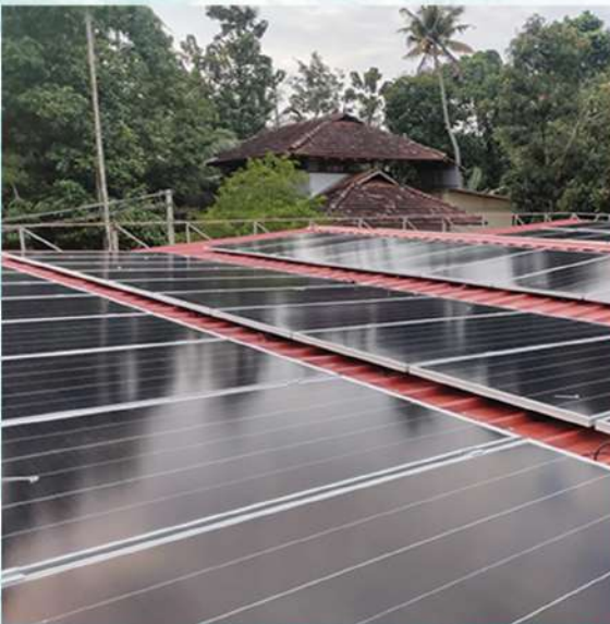
25 kW AT RESIDENCE OF RADHAKRISHNA MENON THRIKODITHANAM
