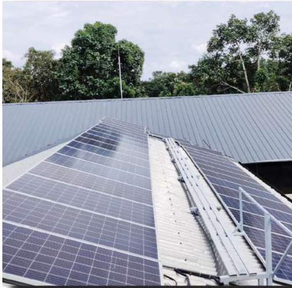
10 kW ON-GRID AT ST JOSEPH PROVINCIAL HOUSE KOTTAYAM
