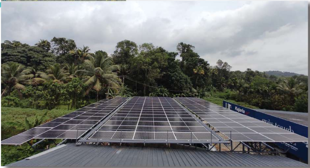
120 kW AT PAITAKULAM MARBLES & GRANITES, KOOHATTUKULAM, KOTHAMANGALAM
