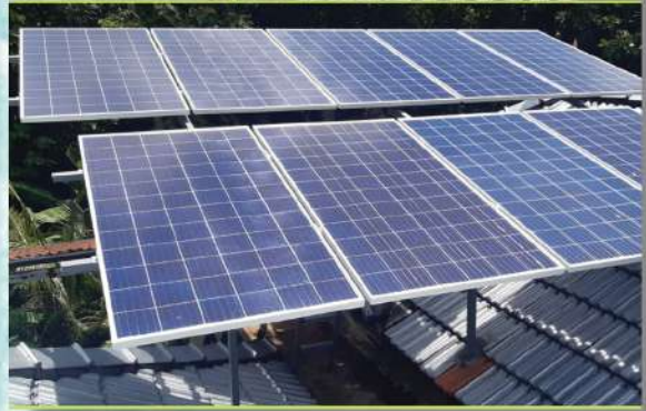
3 kW ON-GRID S S AT THE RESIDENCE OF ROY VARGHESE, PANDALAM
