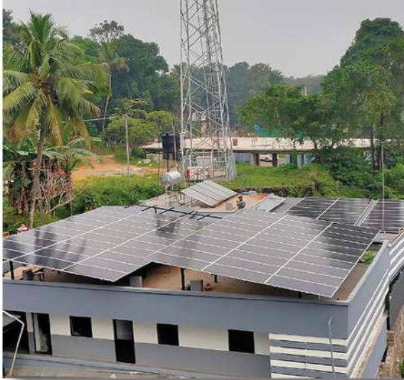
60 kW AT NANGELI AYURVEDA HOSPITAL, KOTHAMANGALAM
