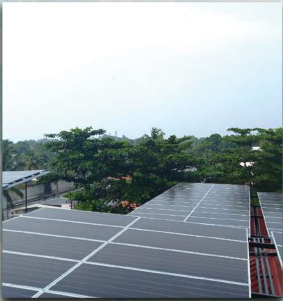
60 kW AT UDAYAGIRI HOSPITAL, CHANGANACHERRY
