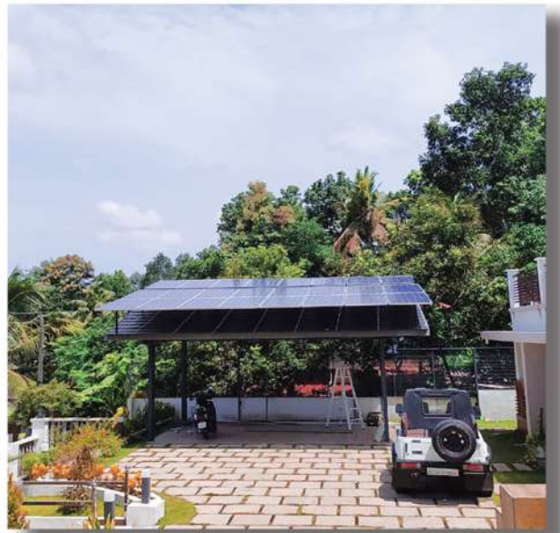
8 kW ON-GRID SOLAR SYSTEM AT KANNANCHIRA , THENGANA
