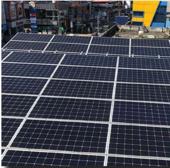
25 kW ON-GRID AT KOHINOOR CHANGANACHERRY
