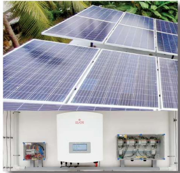
25 kW ON-GRID AT LALGY ENTERPRISES, THIRUVALLA
