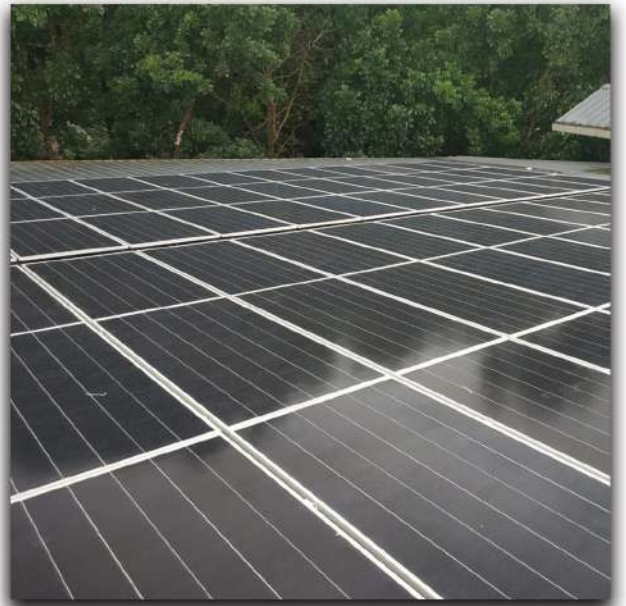
30 kW ON-GRID AT ALLOVEDA HEALTH CARE PERUMPAVOOR, ALUVA
