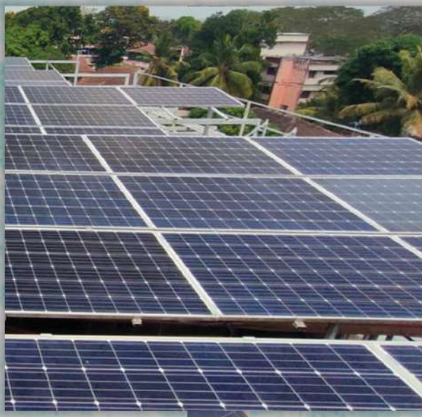
30 kW ON-GRID AT UNIQUE ENTERPRISES THIRUVALLA
