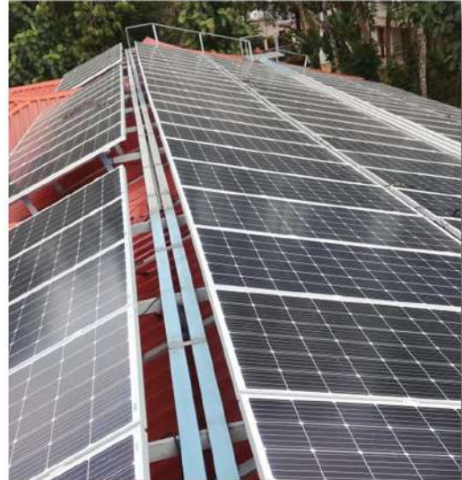
40 kW ON-GRID AT THE RESIDENCE OF SABU T , KOZHENCHERY
