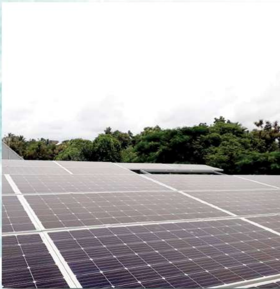
32 kW ON-GRID AT THE RESIDENCE OF MIDHUN, THRISSUR
